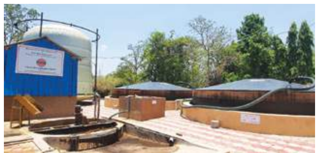
Cattle dung-based Biogas plant at Betul, Madhya Pradesh
