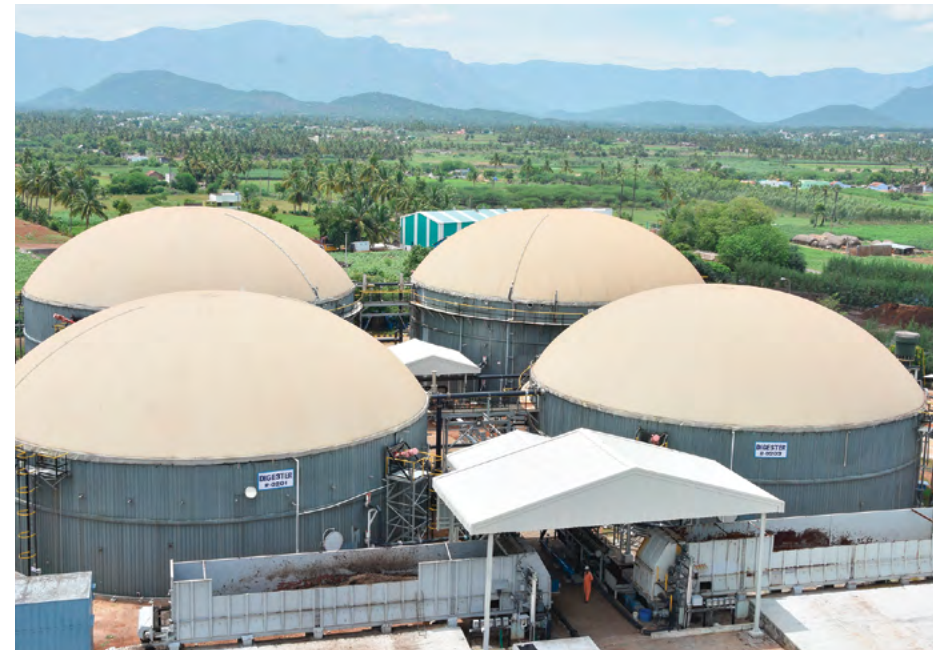
Compressed Biogas Plant (CBG) at Namakkal, Tamil Nadu
