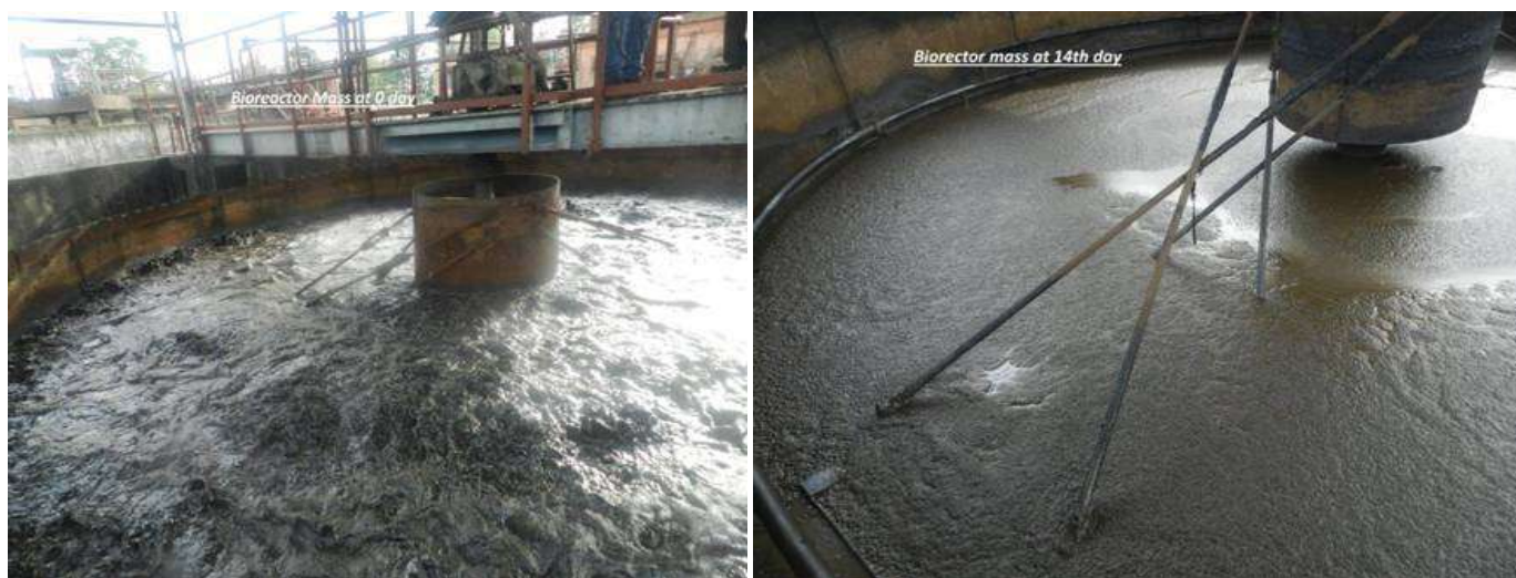
Bio-remediation facility of BGR
