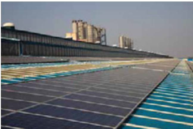
Off-grid solar power plant at IndianOil's Panipat Refinery stands as a testimony to Corporation's commitment to energy transition with an aim to increase its renewable energy capacity to 260 MW by 2020.
