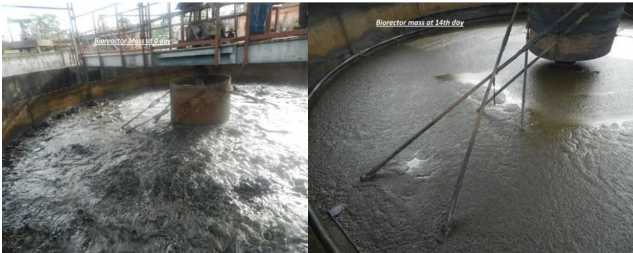
BIO-REMEDIATION FACILITY OF BGR
