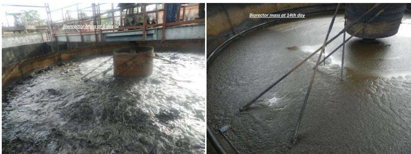
Bio-remediation facility of BGR
