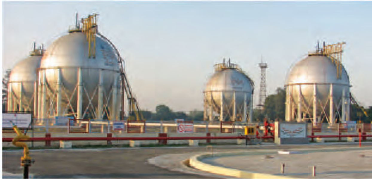
Storage Point at Panipat-Jalandhar LPG Pipeline (PIPL)
