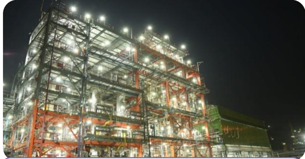
35 TMTPA INDAdept G Plant at Guwahati Refinery
