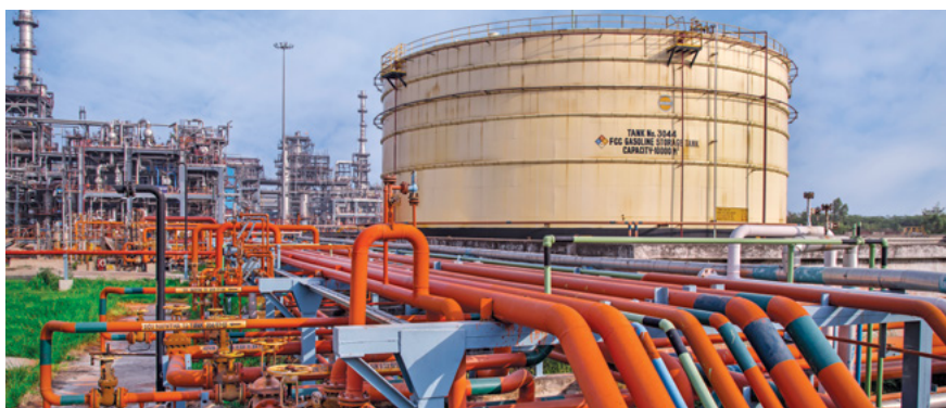
IndianOil owns and operates over 15000 kms of pipelines to reach its energy supplies to the customer touch points
