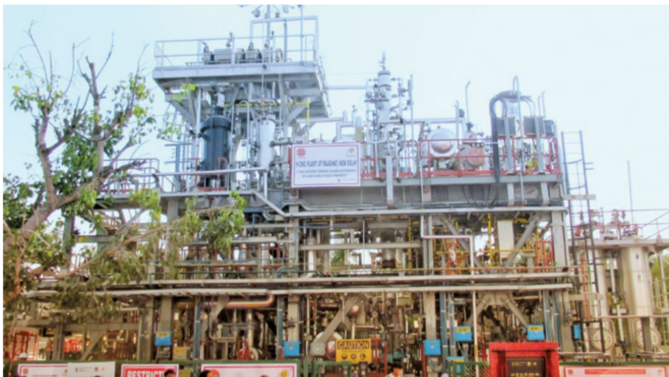
Hydrogen CNG plant at Rajghat, New Delhi
