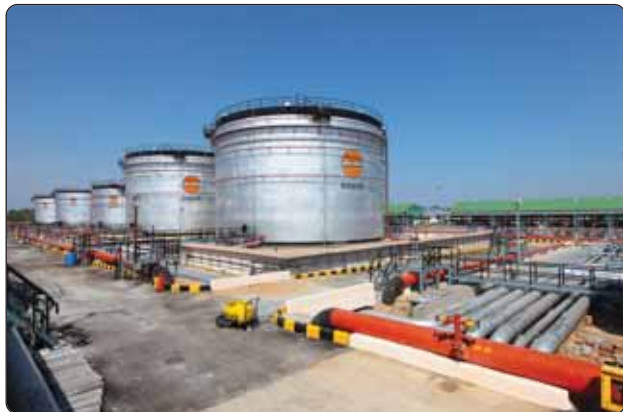
IndianOil's 'smart terminal' at Chittoor in Andhra Pradesh.
