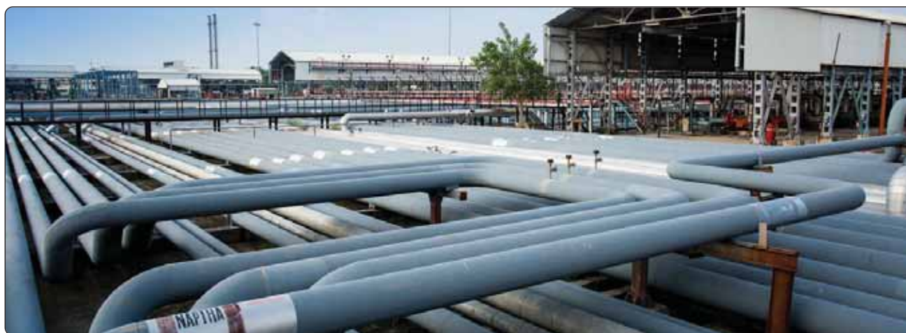
Network of product pipelines at an IndianOil bulk storage terminal.
