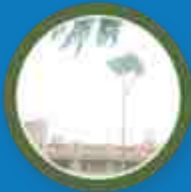
Solar Street Lights
