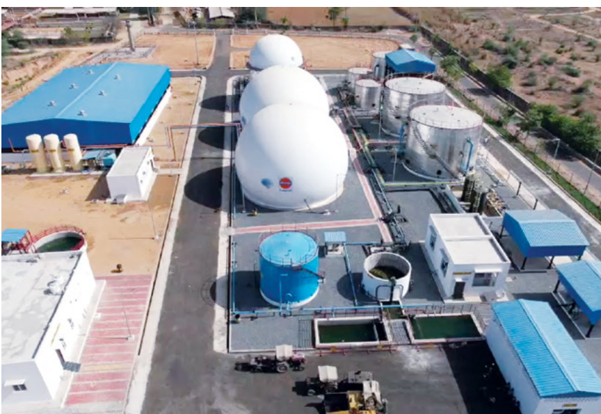
CBG plant at Hingonia, Jaipur
