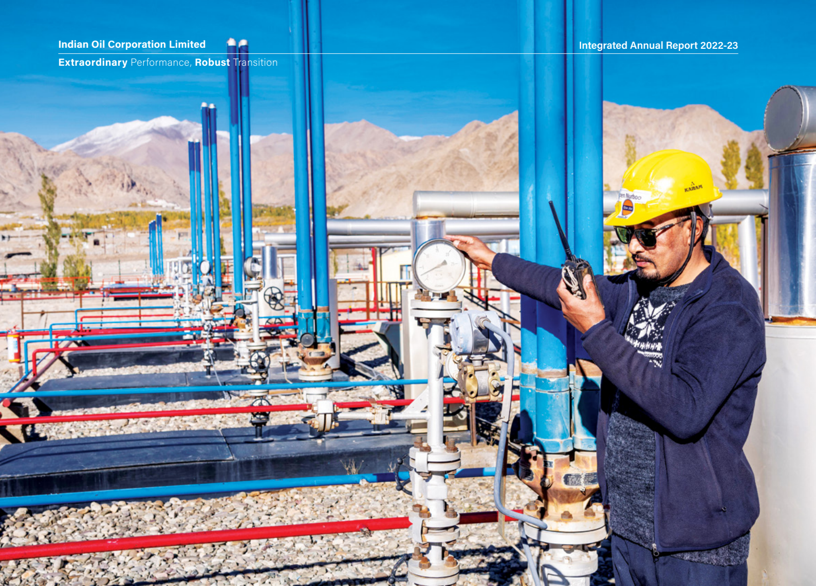
Product pipelines at Leh
