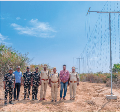
Wildlife initiative involving the installation of Solar Tentacle Fencing for protecting wildlife habitats and avoiding man-animal conflict
