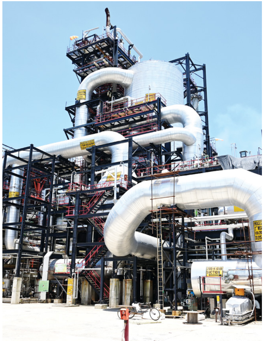
Wet Sulphuric Acid Plant at Haldia Refinery
