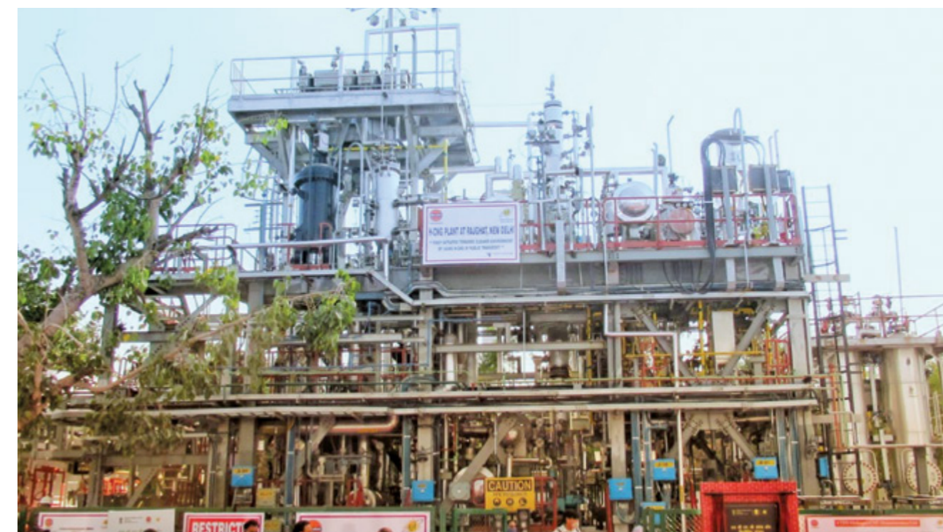
Hydrogen CNG plant at Rajghat, New Delhi
