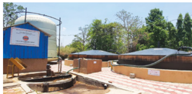
Cattle dung-based Biogas plant at Betul, Madhya Pradesh
