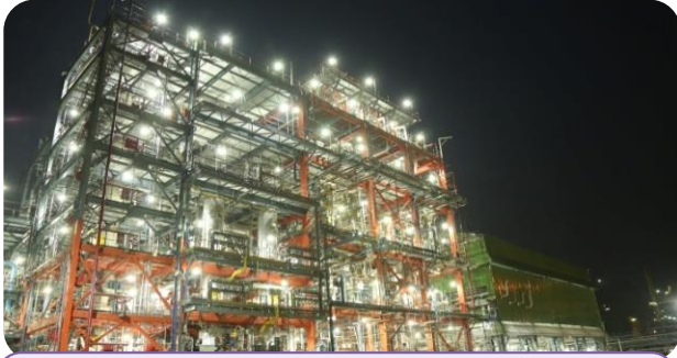
35 TMTPA INDAdept G Plant at Guwahati Refinery
