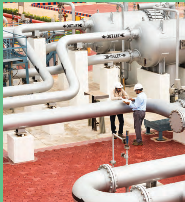
A pipeline terminal on the Paradip-Raipur-Ranchi product pipeline.
