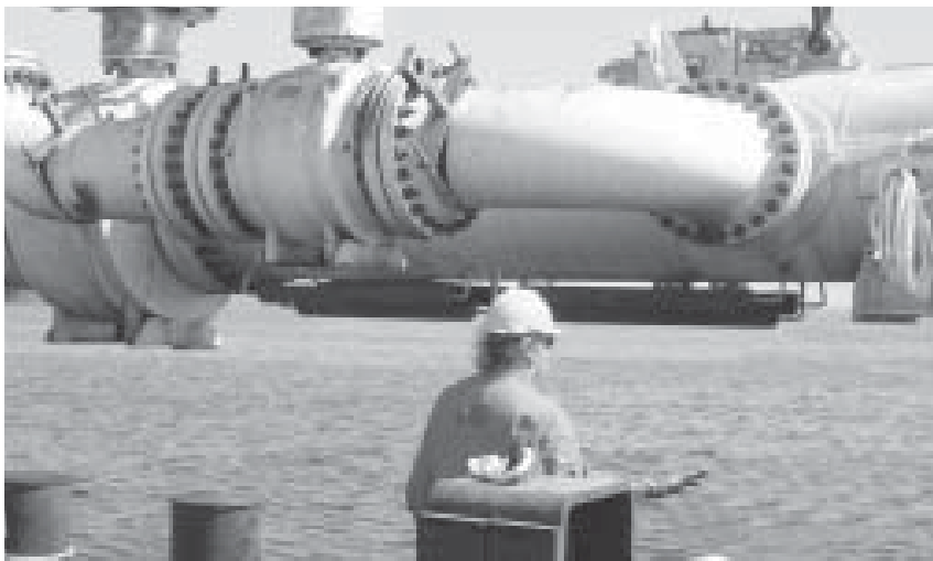
The Paradip-Haldia crude oil pipeline.
