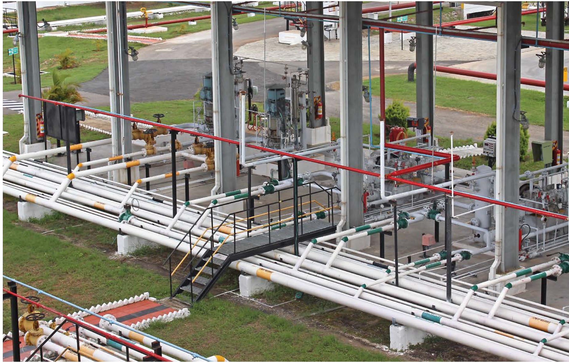
LPG pump and compressor house at the Mysore bottling plant
