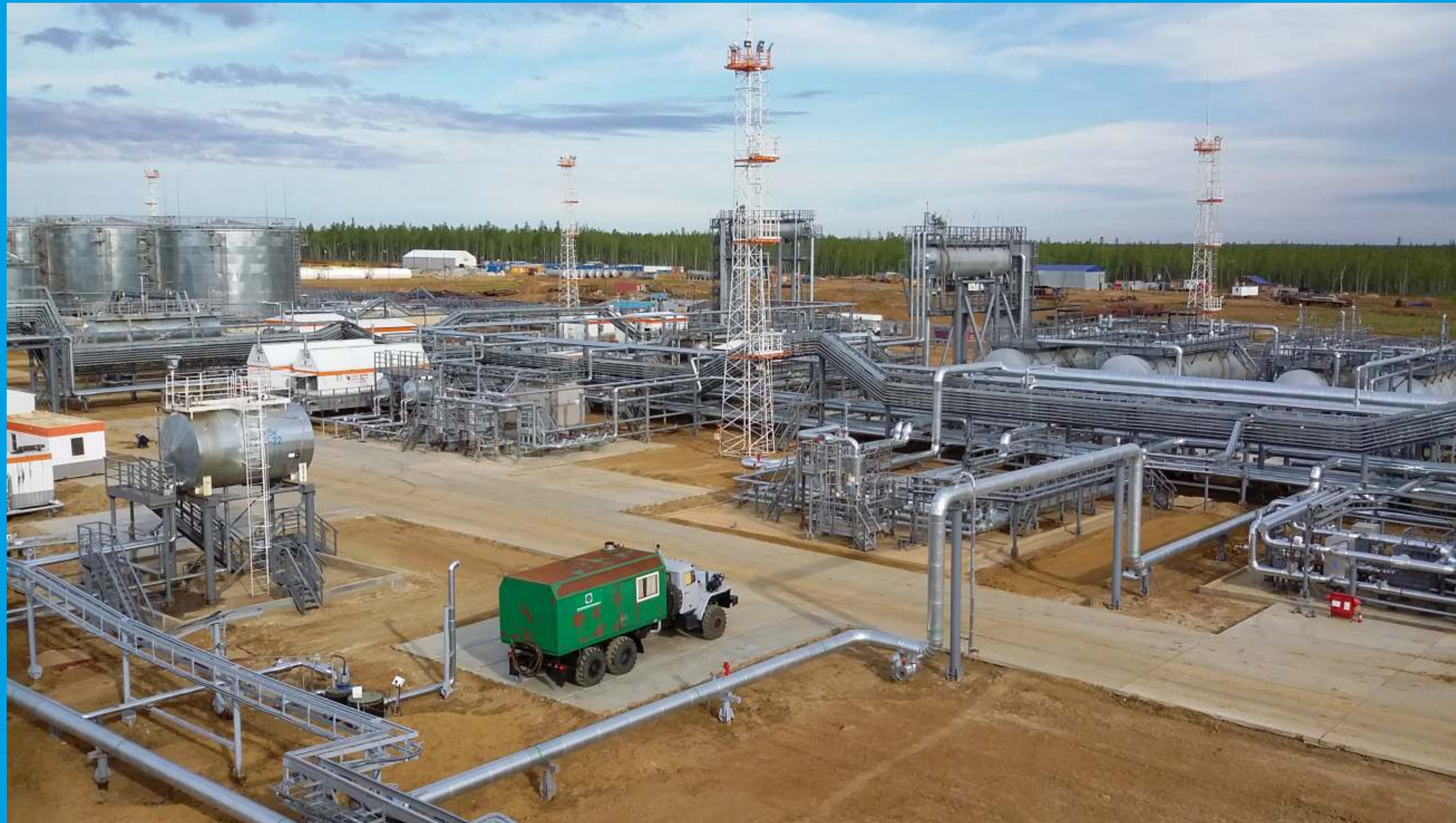
Oil Treatment facility at TAAS asset, Russia IndianOil, OIL and BPRL, through a Special Purpose Vehicle (SPV) TAAS India Pte. Ltd., acquired 29.9% stake in TYNGD from Rosneft. IndianOil's share of net production from this asset is ~10,500 bopd.
