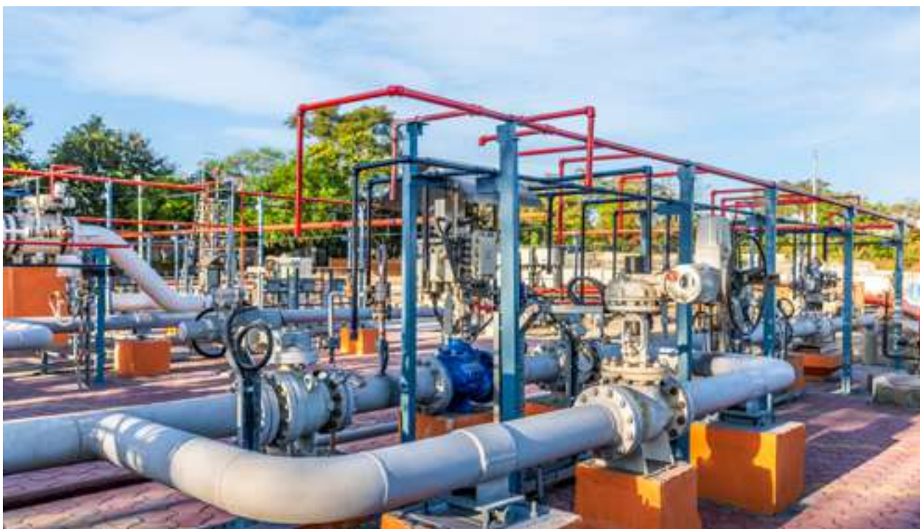
Mundra Panipat Pipeline Hub
