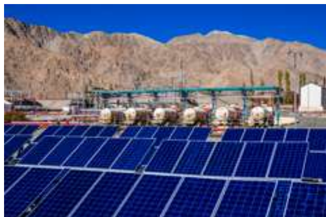
Solar Powered Indane Bottling Plant, Leh
