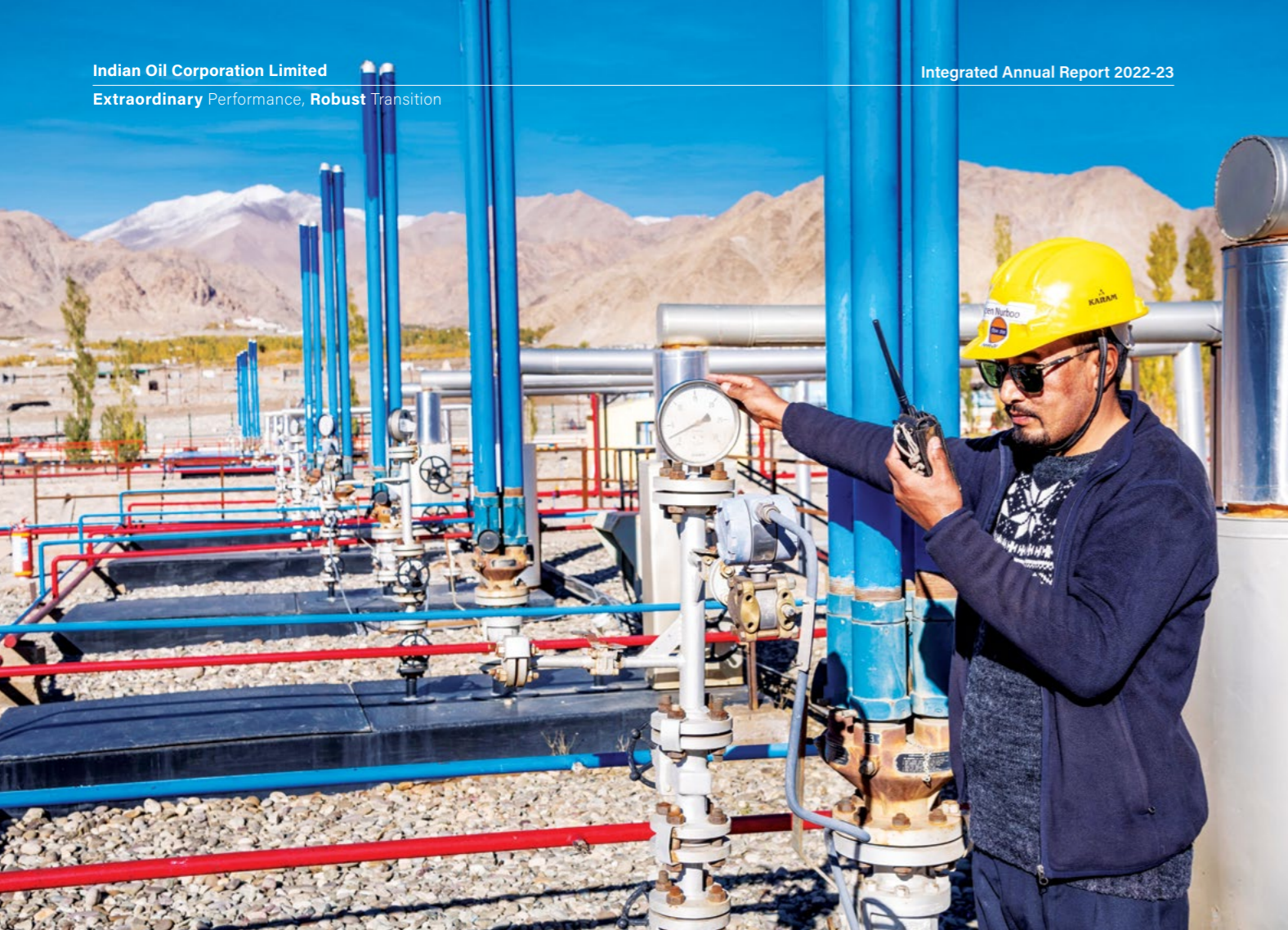
Product pipelines at Leh
