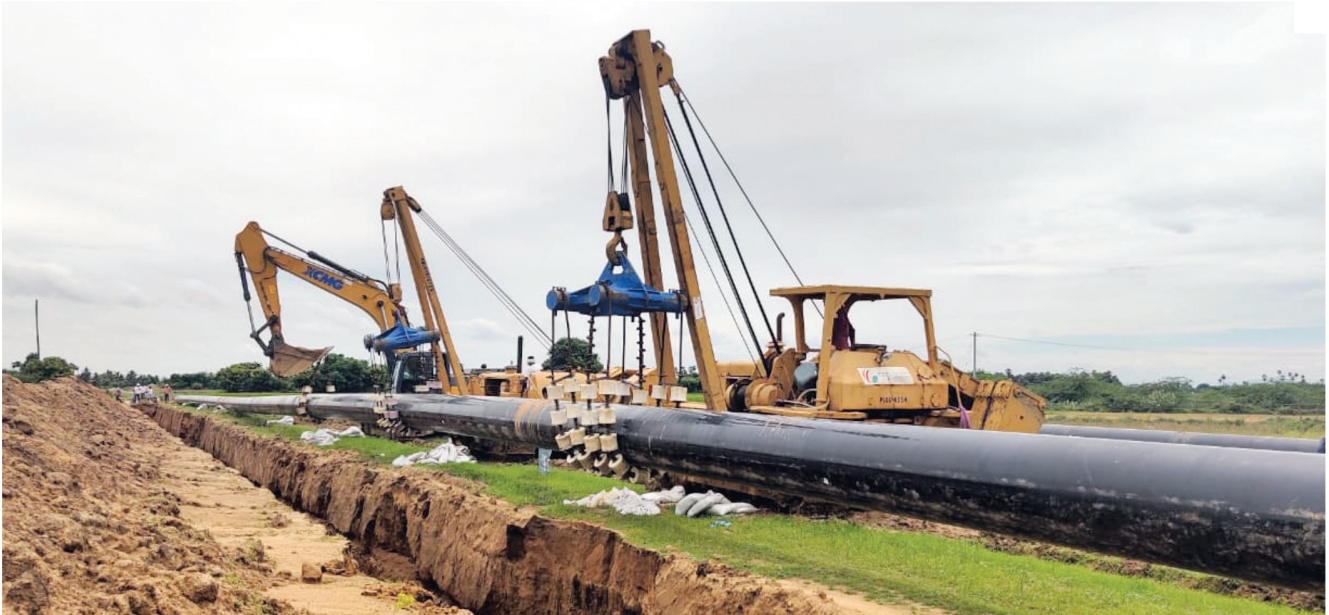
IndianOil's Pipeline infrastructure has expanded with the completion of the 1200 Km-long Paradip-Hyderabad product Pipeline
