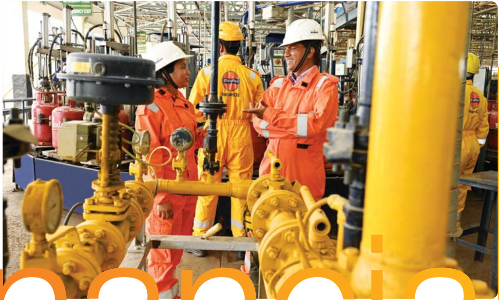
IndianOil LPG Bottling plant in Digboi, Assam
