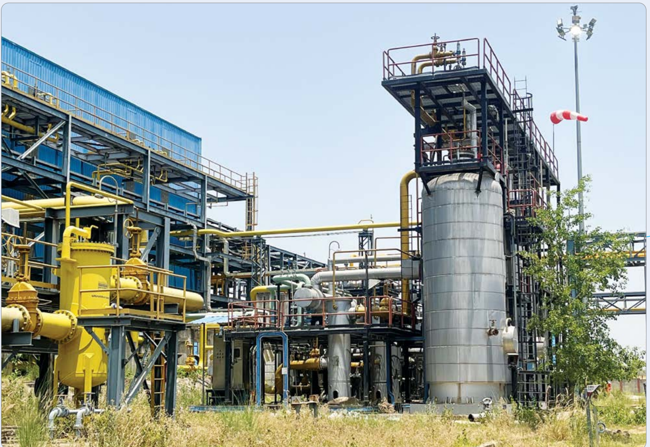
▶ Gas Collecting Station (GCS), Bokaro- a major production installation for processing of Coal Bed Methane gas
