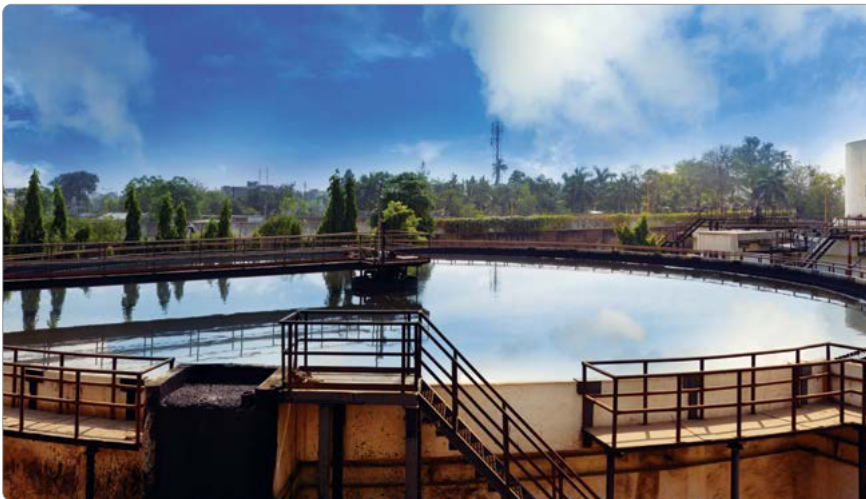
▶ Clarifier at Gujarat Refinery for treatment of sewage waste for reusing water
