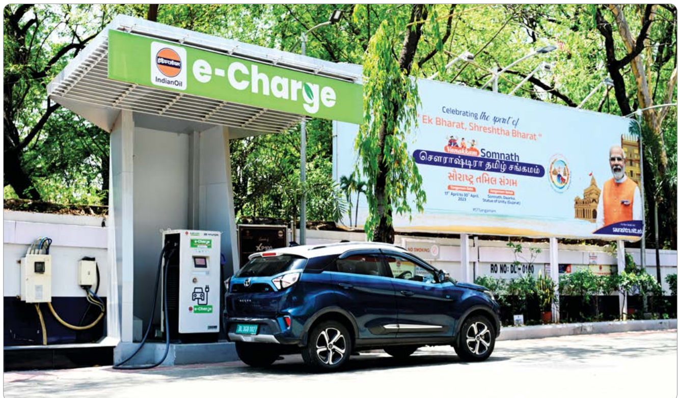
▶ EV Charging Facility at IndianOil fuel station
