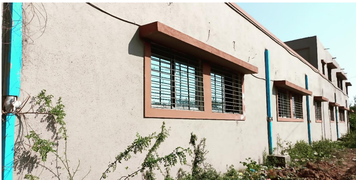
Figure 5: Rainwater Harvesting setup installed in a school in Vadodara
