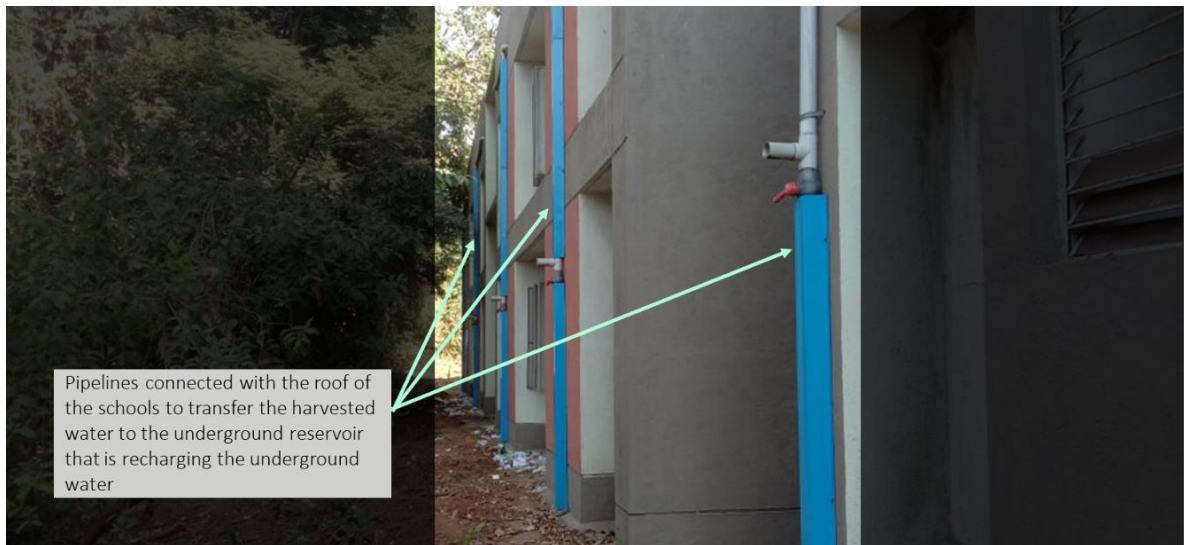
Figure 43: A rainwater harvesting unit installed in a primary school in Vadodara
