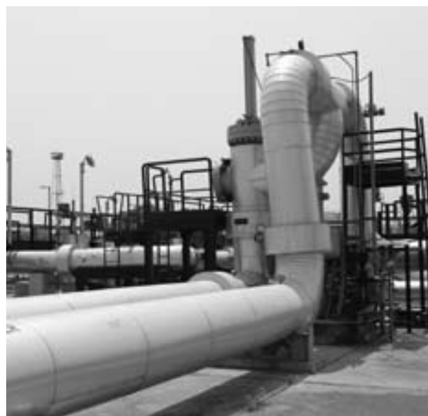
IndianOil Paradip-Haldia-Barauni Pipeline
