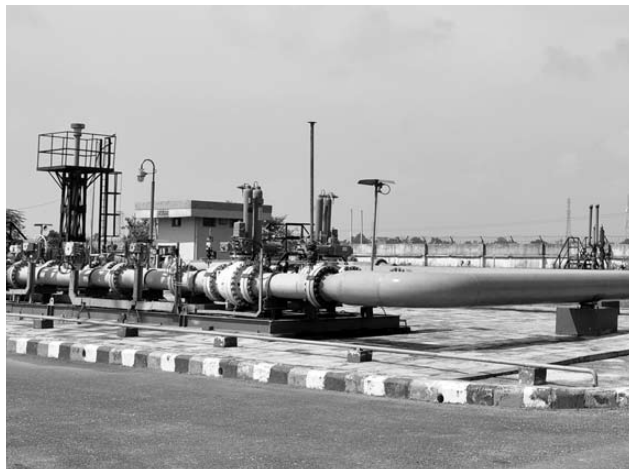
Dadri gas pipeline
