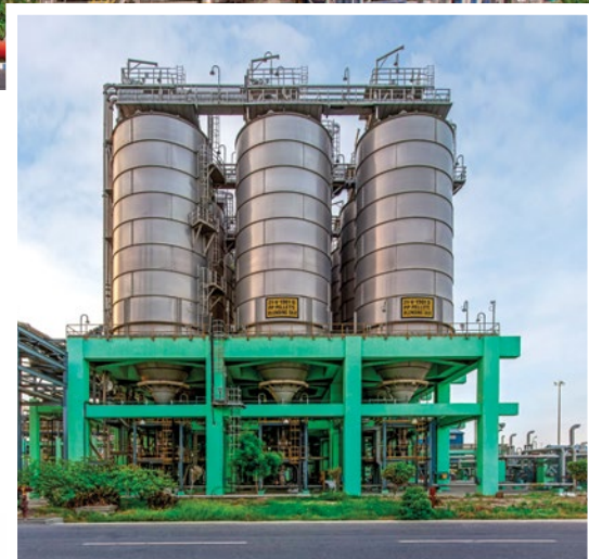
PP Unit (PP Pellets Blending Silo)
