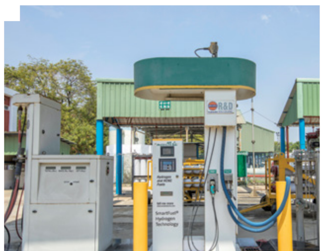
Smart Fuel Hydrogen Technology Station installed at IndianOil R&D Centre at Faridabad, Haryana
