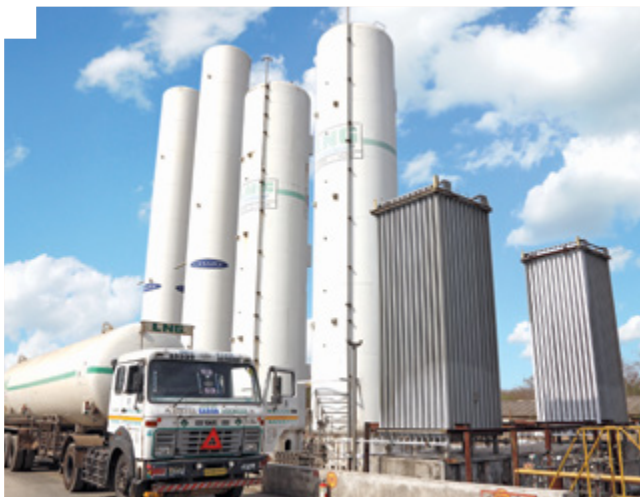
IndianOil, through its Joint Venture Company, IndianOil LNG Pvt. Ltd., has developed a 5-million metric tonnes per annum (MMTPA) capacity Liquefied Natural Gas (LNG) Terminal at Kamarajar Port, Ennore in Tamil Naidu
