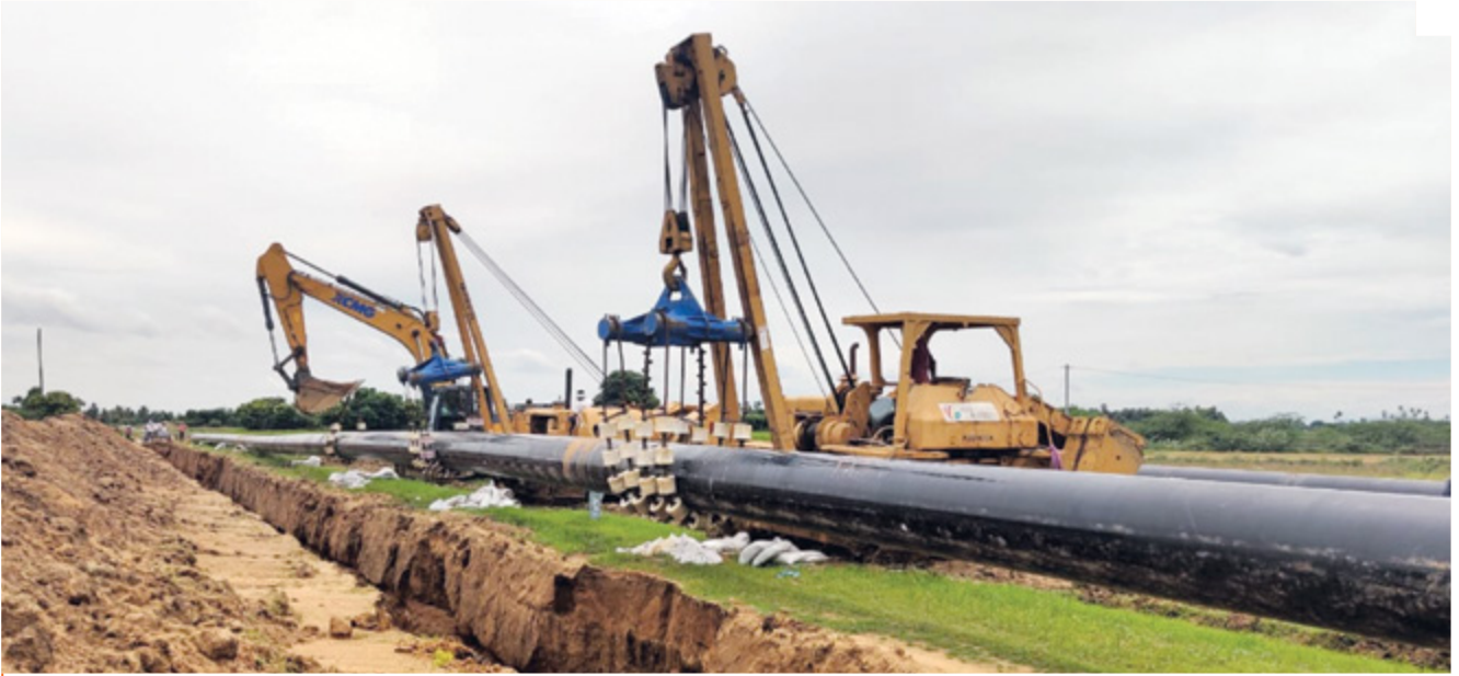
IndianOil's Pipeline infrastructure has expanded with the completion of the 1200 Km-long Paradip-Hyderabad product Pipeline
